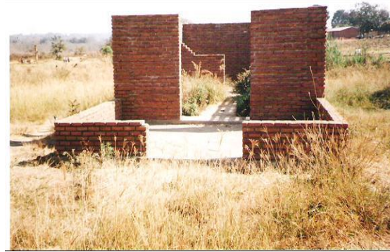
Figure 4.6 Failure: Uncompleted Maize Mill House at the same site as (4.5) Source: Field Photographs
