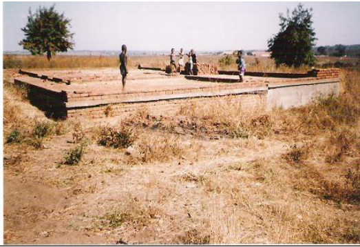
Figure 4.5 Cheated: Uncompleted ECD centre foundation in Phwetekere at which a CBO spent MK909387.55 (US$6495.63). Source: Field Photographs
